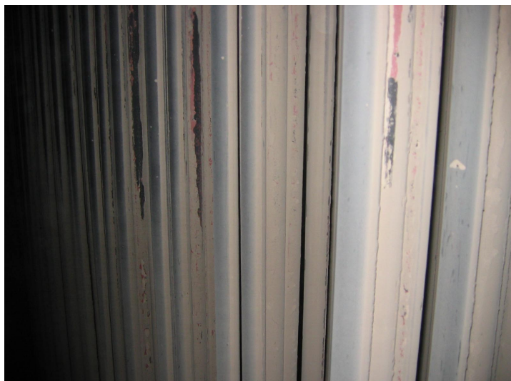
Fig. 4. The superheater I tubes in Block No. 8 at the Eesti PP
